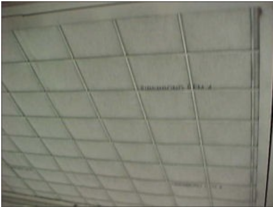
DFM 4 media utilized as a ceiling filter in a downdraft paint booth.
